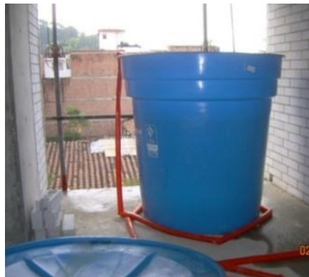
Photo 1. Storage tank. Source: Pineda, E. (2015).
